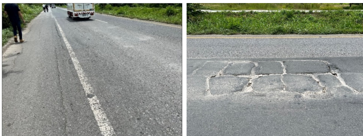
Figure 3 Pavement distresses along highway No. 117.
